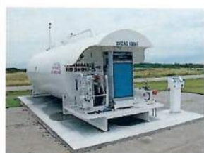
8,000 Gallon Tank with a Dispenser Style Fueling System
