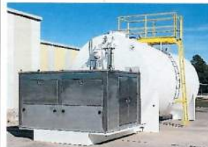
12k – Stainless Steel Enclosure Cabinet and Side Mount Platform-Ladder
