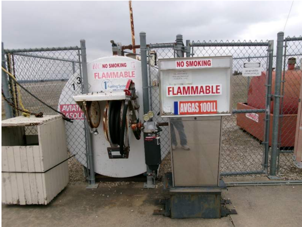
Existing AvGas Dispenser
