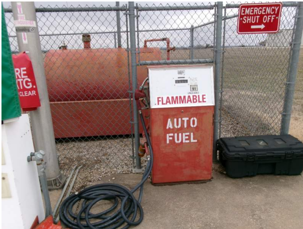
Existing MoGas Dispenser
