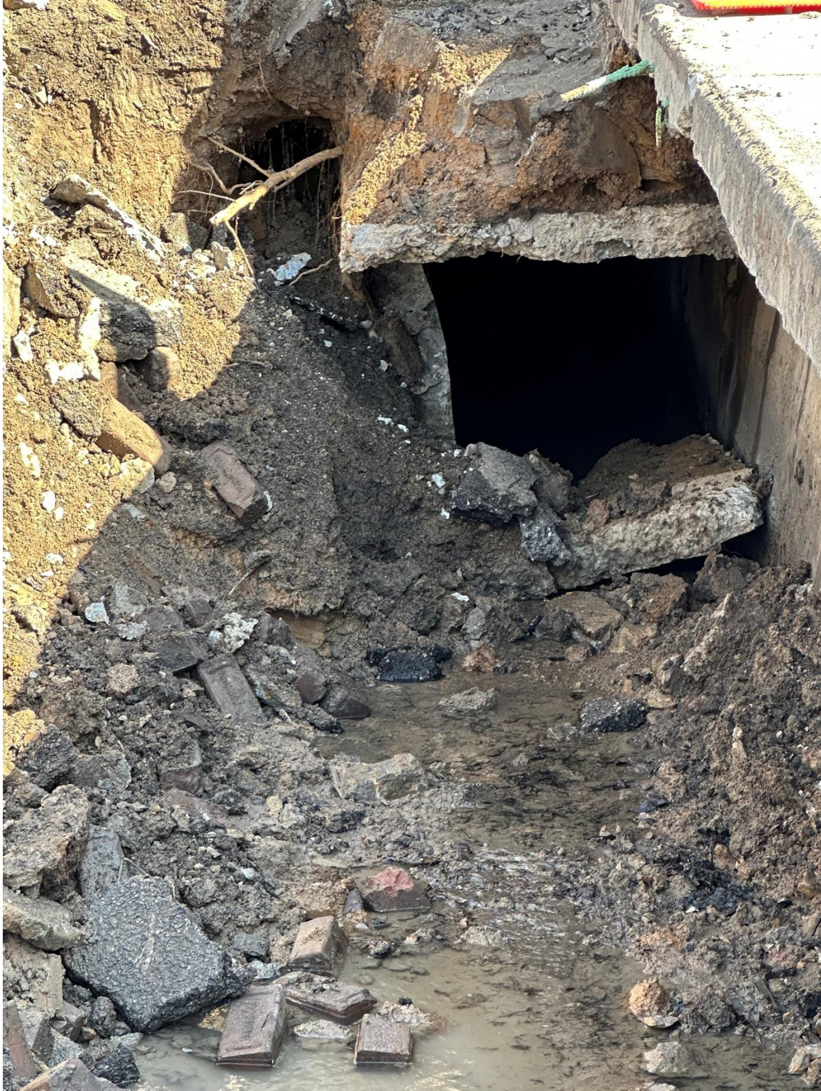
(Looking north towards 10 th Ave, wall along west side giving way near floor) (east side wall looked to be leaning also) (circa 1900-1920 from plan archives) (Pictures 2026.03.30)
