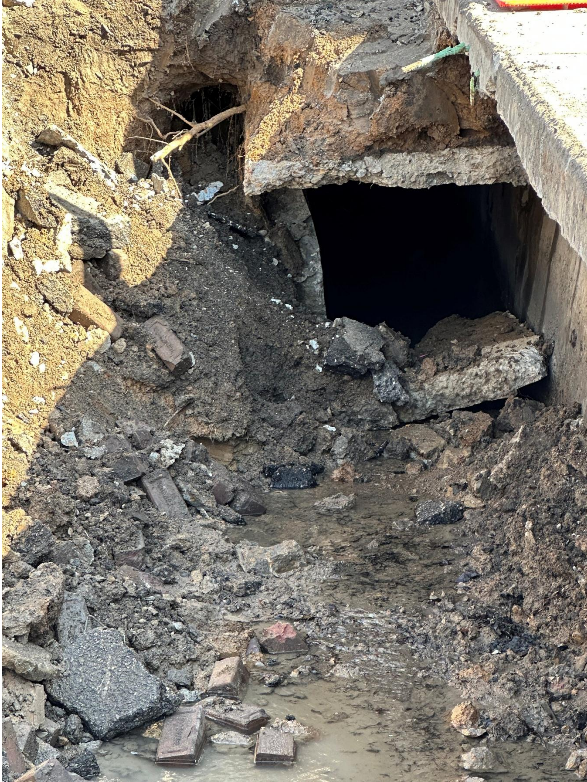
(Looking north towards 10 th Ave, wall along west side giving way near floor) (east side wall looked to be leaning also) (no sign of rebar in walls, consistent with detail from plans, circa 1900-1920) (Pictures 2026.03.30)
