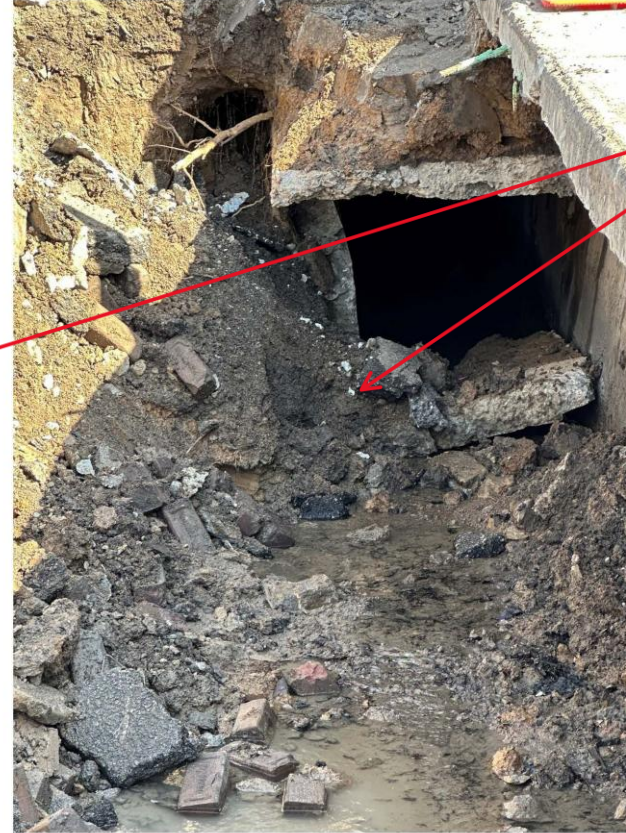
(Looking north towards 10 th Ave, wall along west side giving way near floor) (east side wall looked to be leaning also) (circa 1900-1920 from plan archives) (Pictures 2026.03.30)
