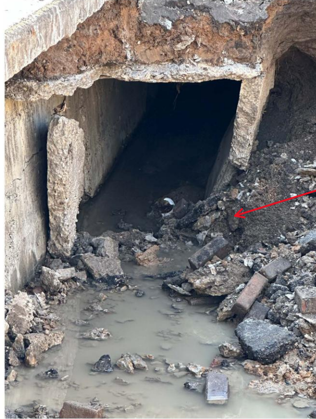
(Looking south toward 9 th Ave, wall along west side giving way near floor) (east side wall looked to be leaning also) (circa 1900-1920 from plan archives) (Pictures 2026.03.30)
