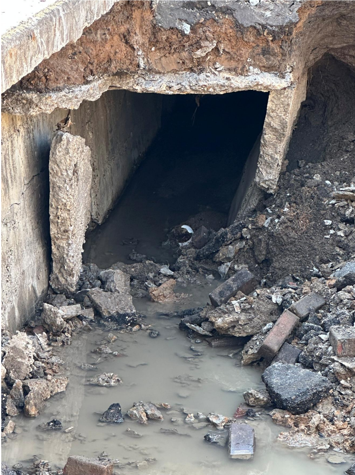
(Looking south toward 9 th Ave, wall along west side giving way near floor) (east side wall looked to be leaning also) (no sign of rebar in walls, consistent with detail from plans, circa 1900-1920) (Pictures 2026.03.30)
