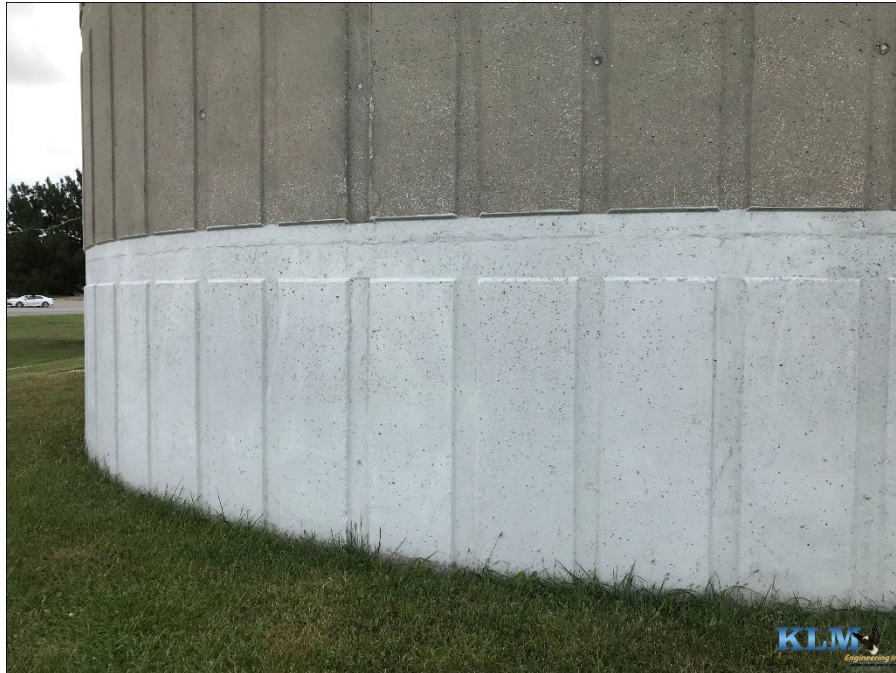
Photo No. 55 Painted over section of base to cover grafitti
