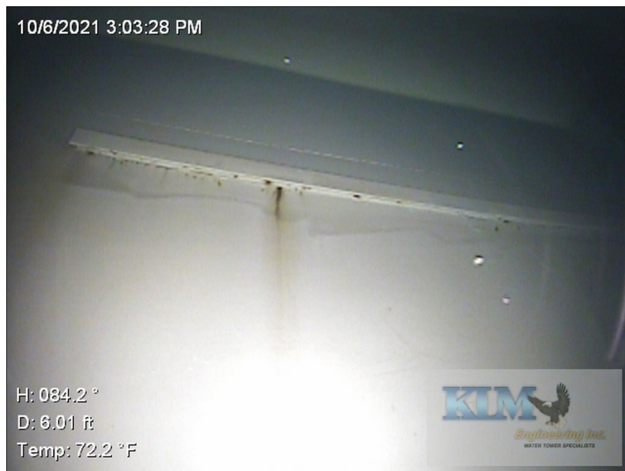
Photo No. 28 Shell condition; Corrosion on bottom of shell erection angle visible
