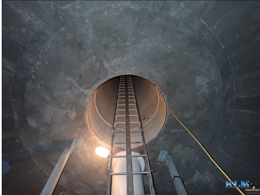
Photo No. 33 Drywell tube and bowl
