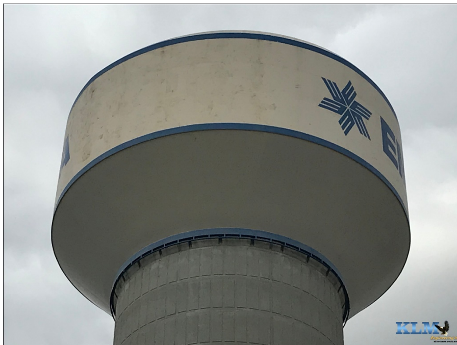
Photo No. 52 Coating condition on shell and bowl
