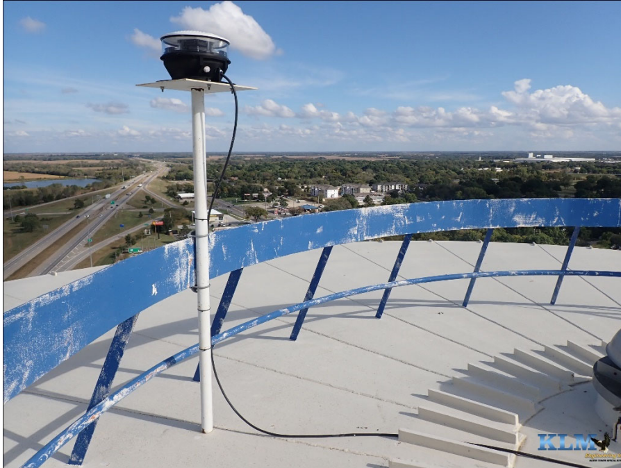
Photo No. 45 Roof handrail and aviation light
