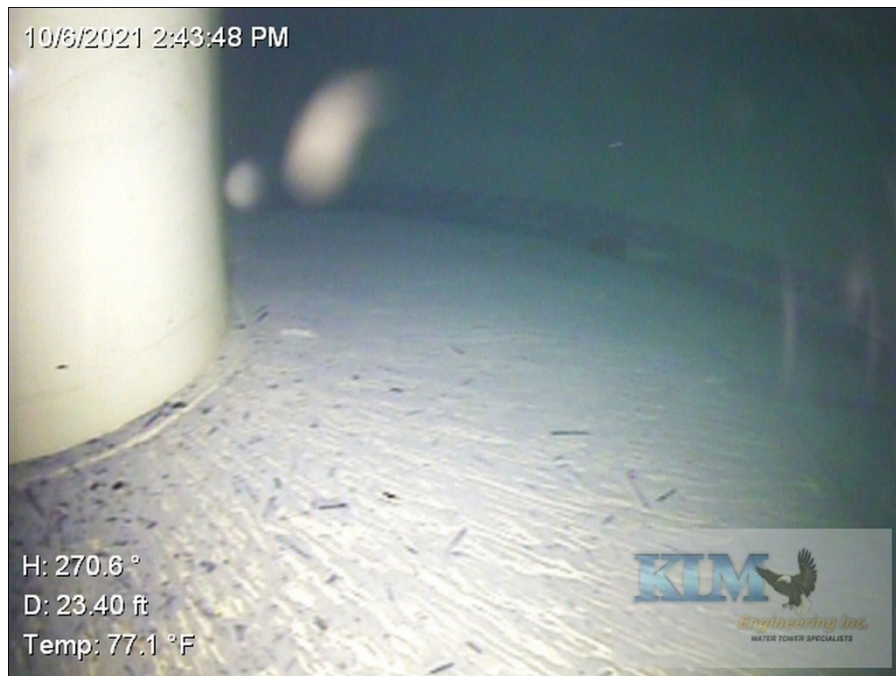
Photo No. 15 Condition of bowl
