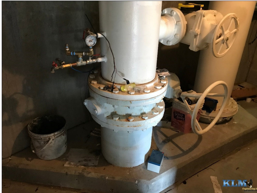
Photo No. 41 Piping in control room
