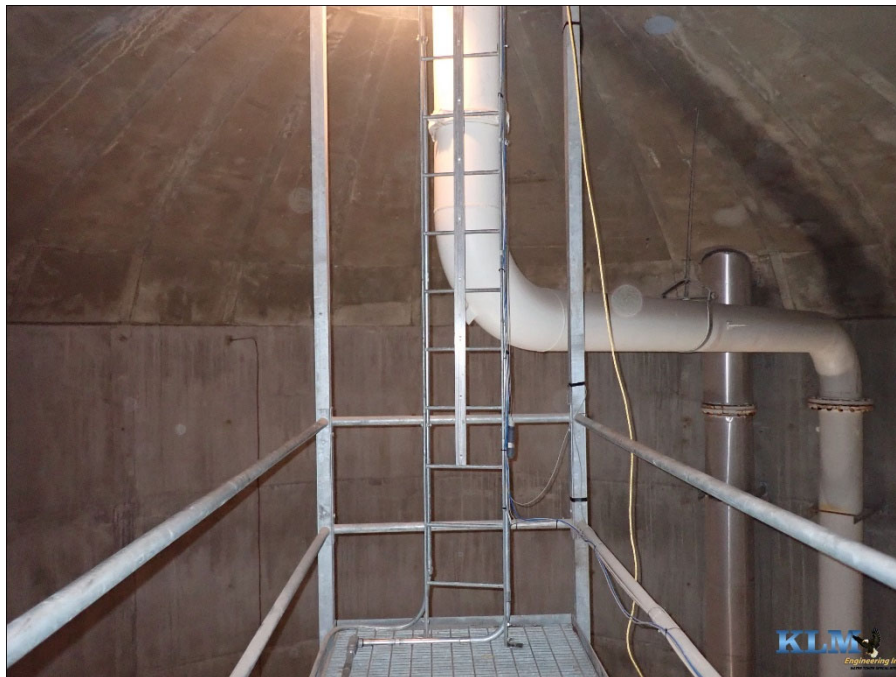
Photo No. 34 Catwalk and piping
