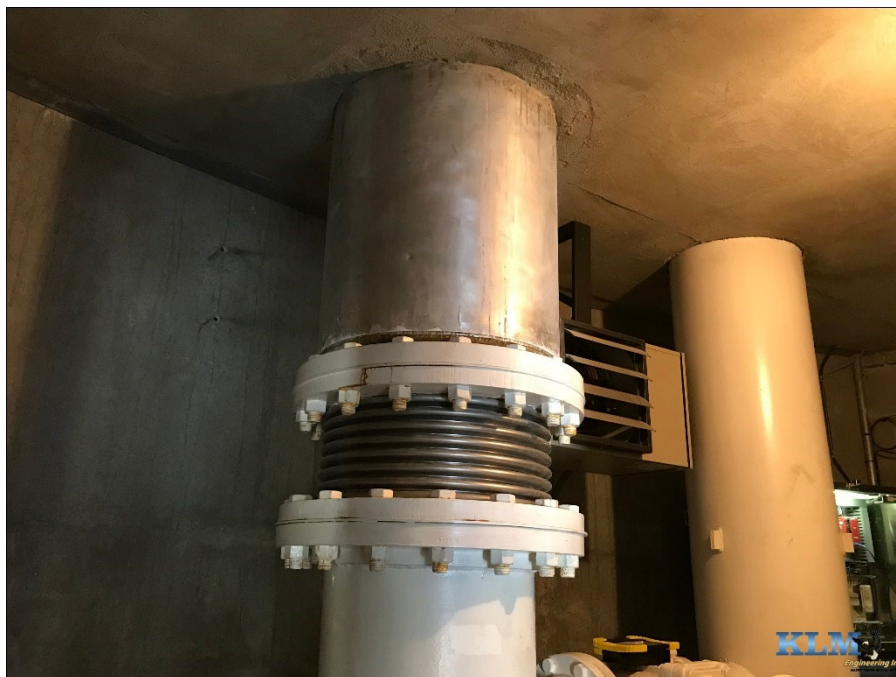
Photo No. 42 Piping in control room; expansion joint shown
