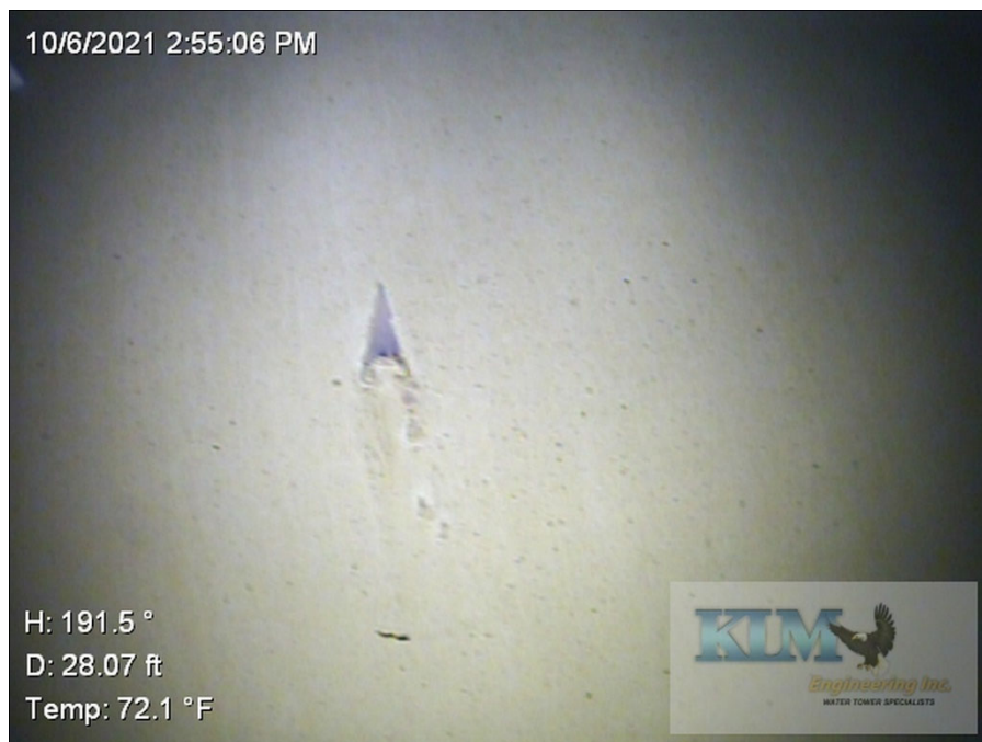
Photo No. 20 Erection scab mark in cone
