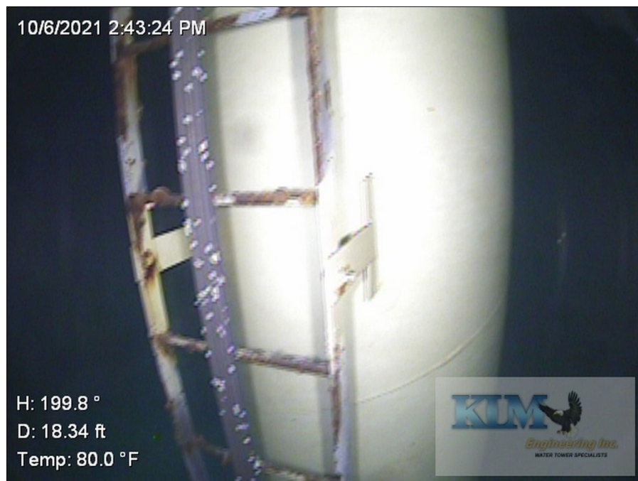
Photo No. 14 Drywell tube and ladder
