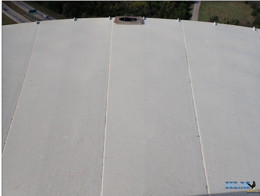
Photo No. 49 Roof coating condition, Note; damaged manway
