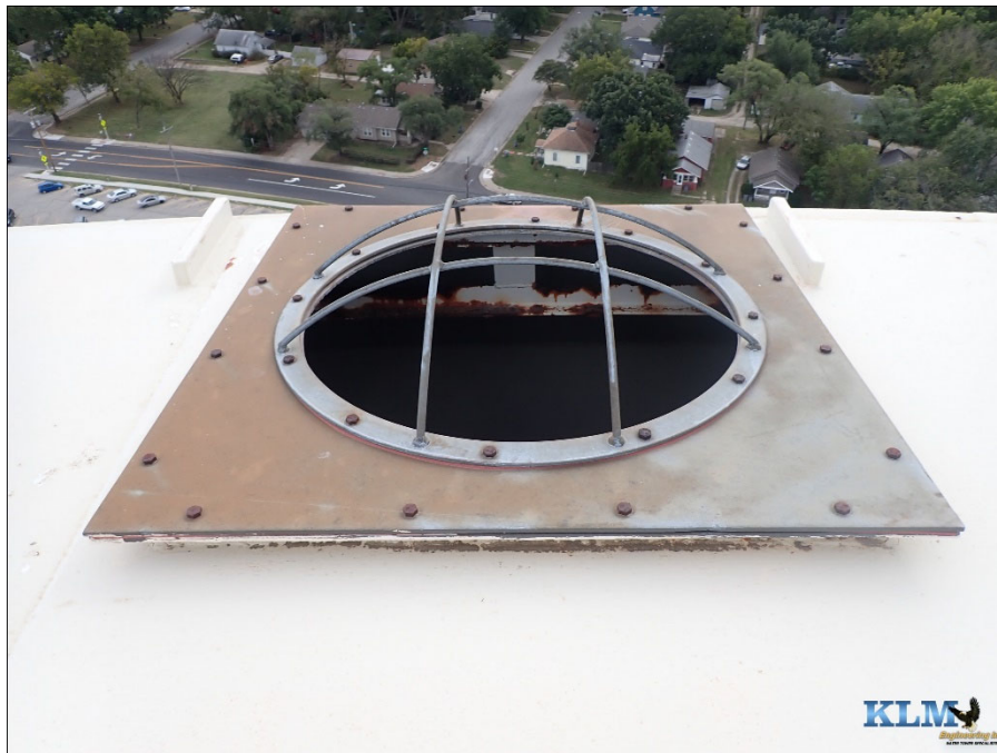
Photo No. 50 Non-compliant, damaged outer access manway
