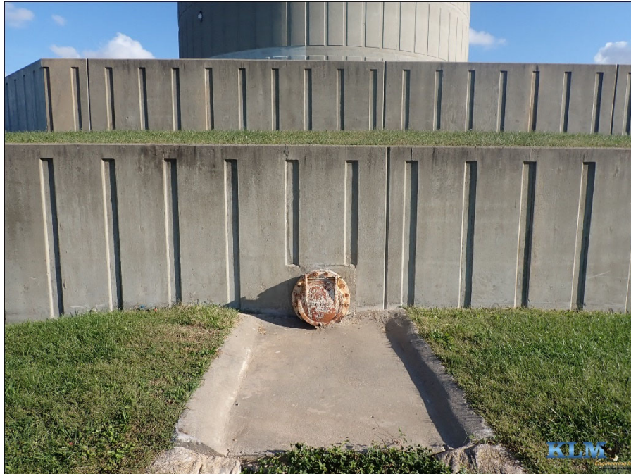
Photo No. 57 Overflow discharge on retaining wall
