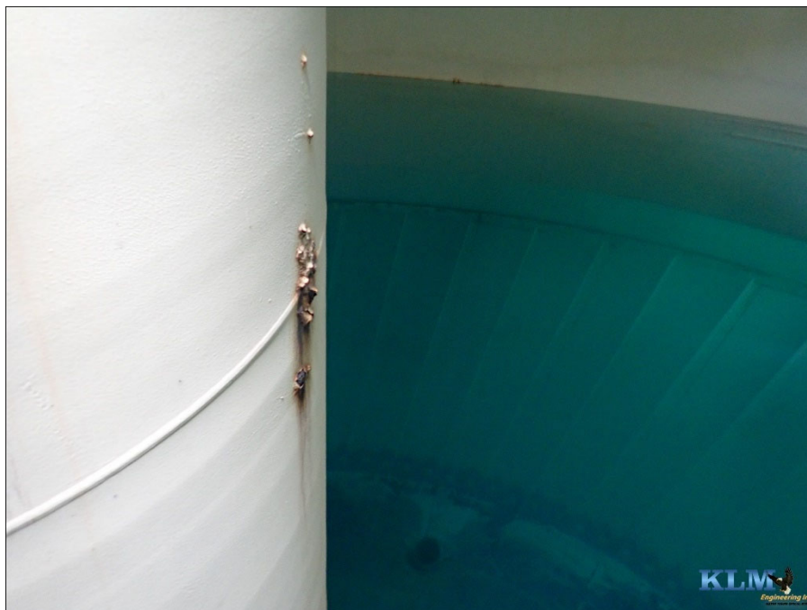
Photo No. 12 Coating failures on drywell tube
