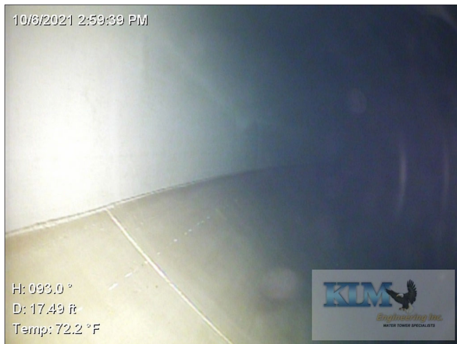
Photo No. 22 Conditions at cone to shell connection
