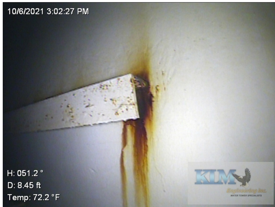
Photo No. 27 Corrosion at shell erection angle
