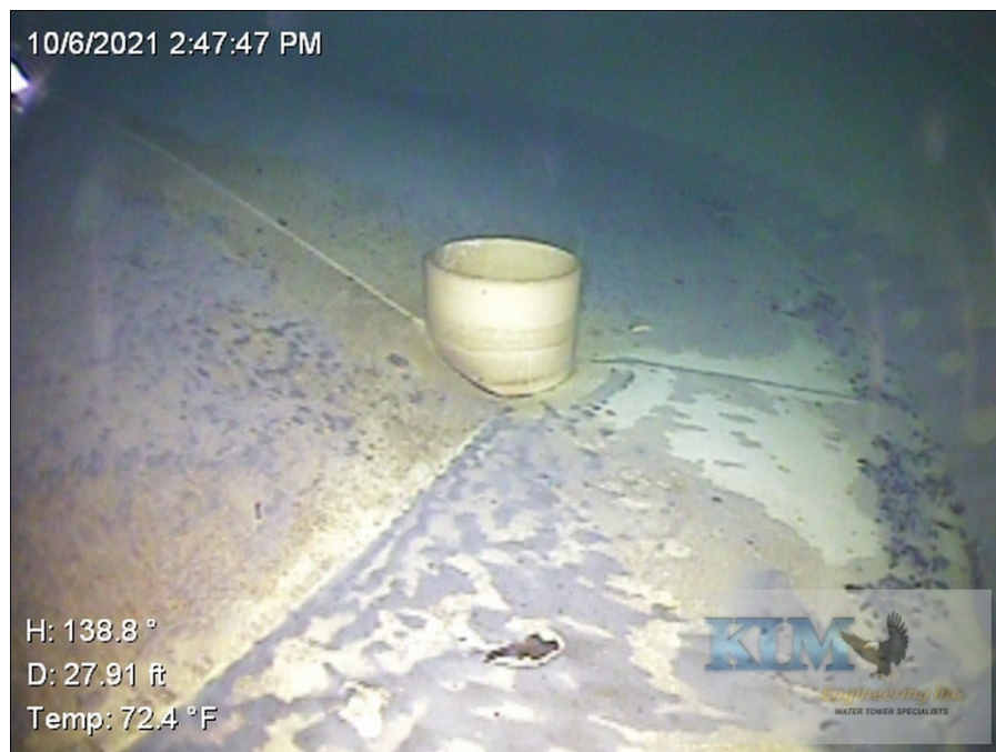
Photo No. 18 Fill pipe and lower bowl
