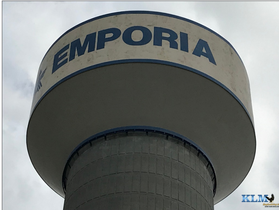
Photo No. 53 Coating condition on shell and bowl
