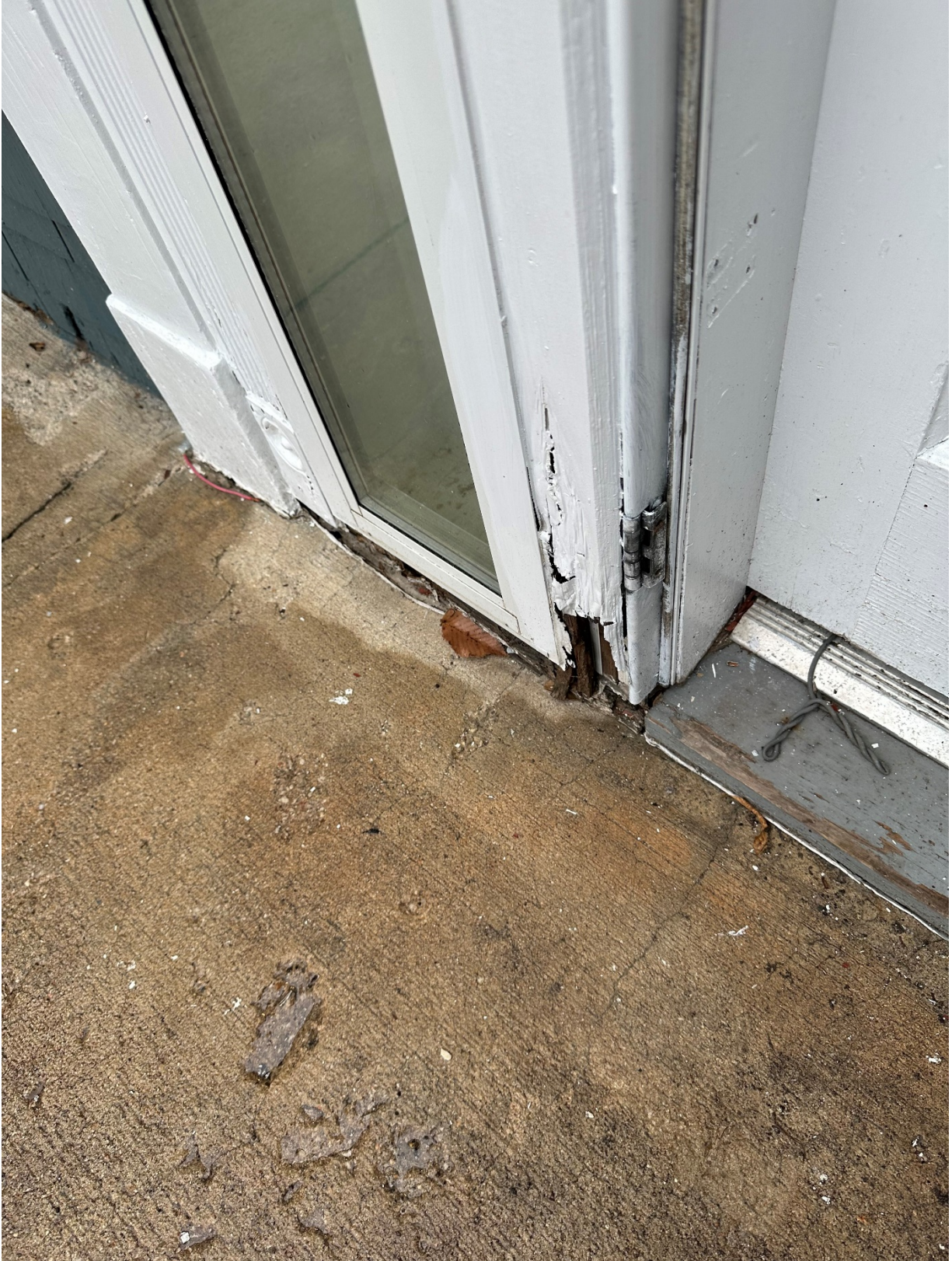
Existing Wood Rot
