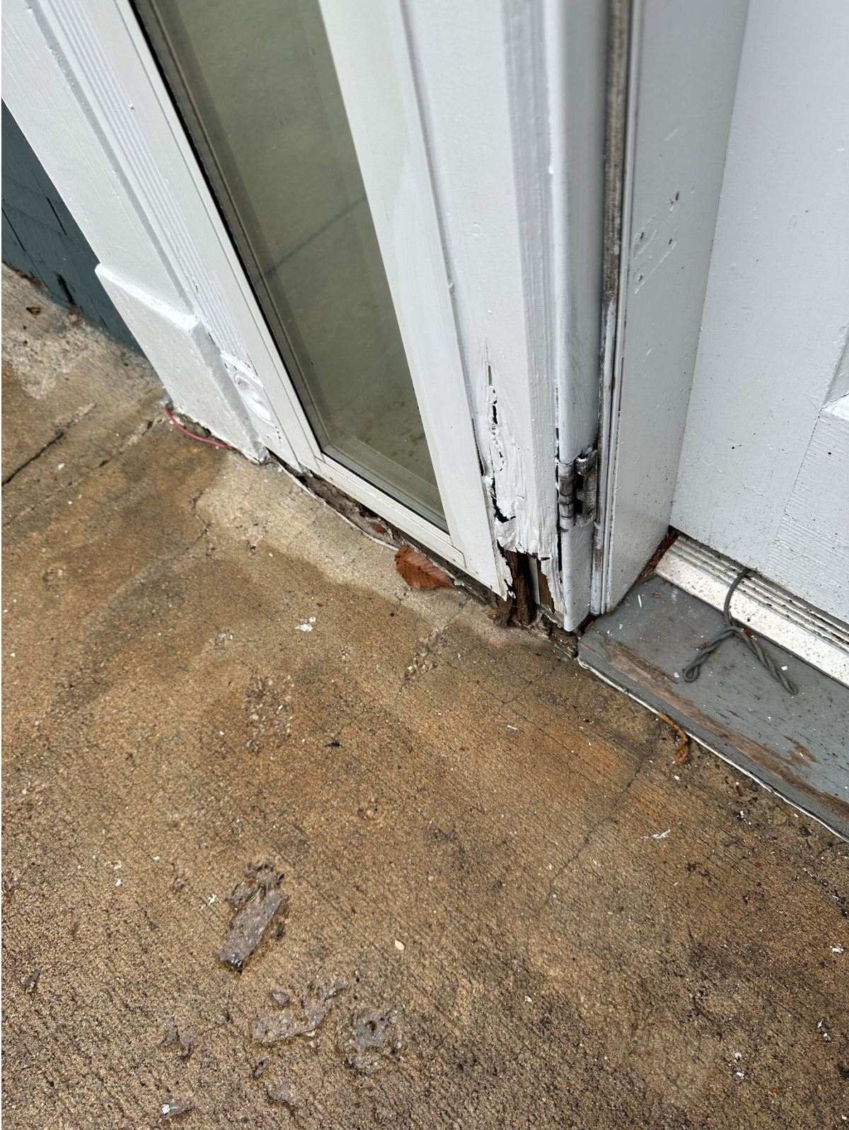
Existing Wood Rot
