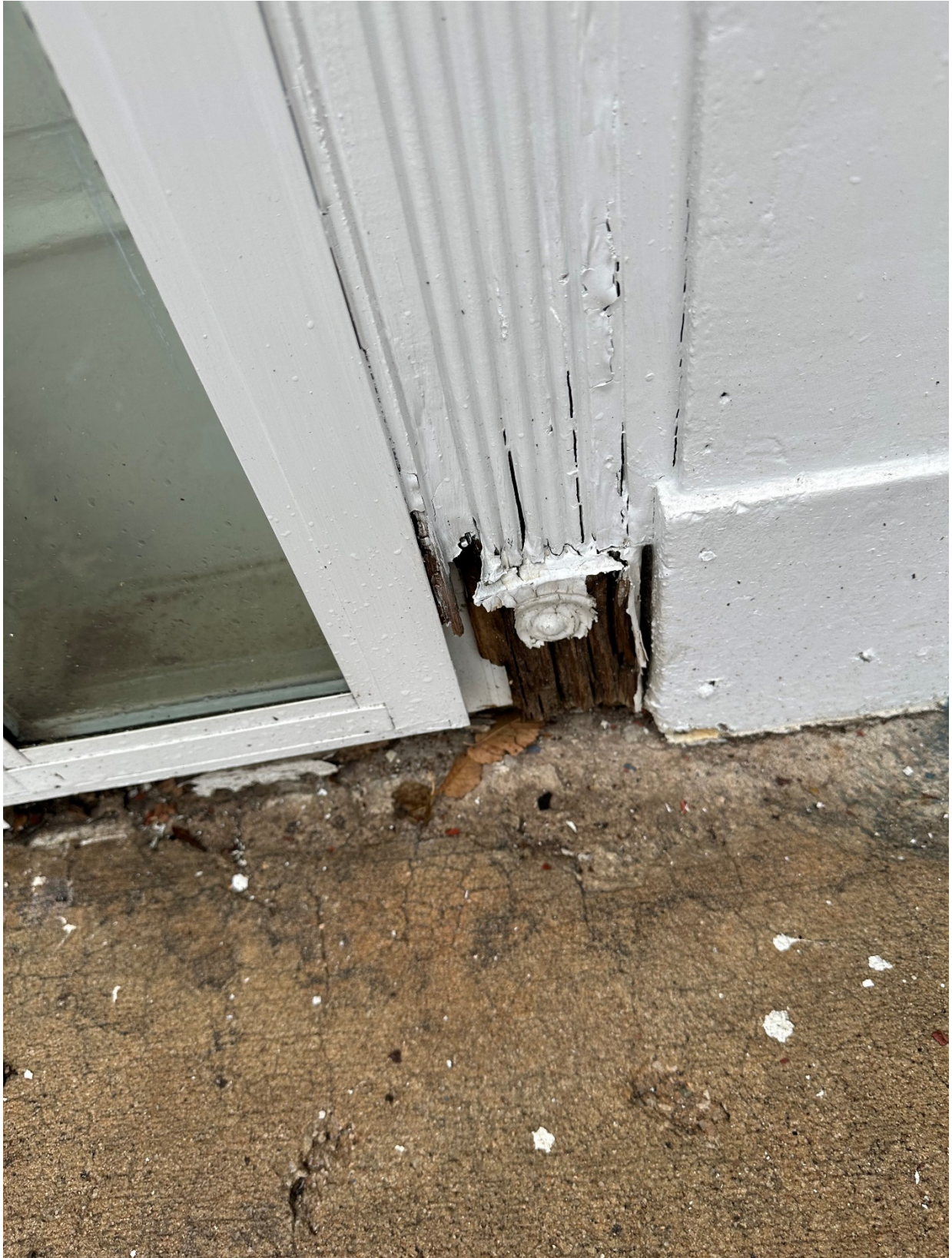
Existing Wood Rot
