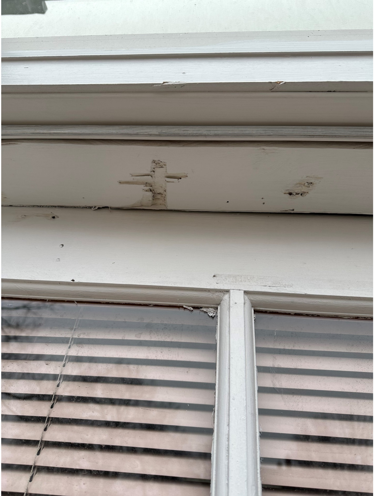
Existing Wood Rot
